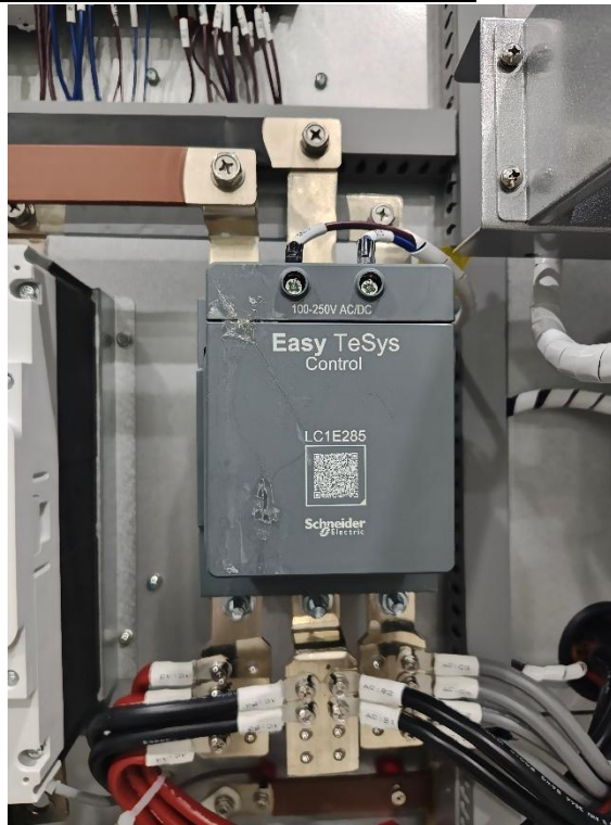
Figure 65 AC contactor KM1
