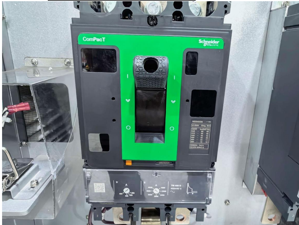
Figure 11 AC circuit breaker QF1
