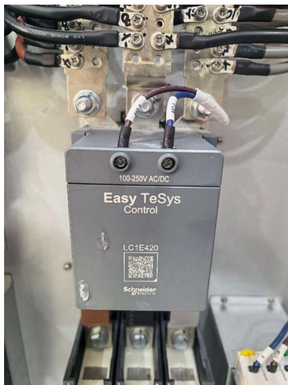
Figure 12 AC contactor KM1
