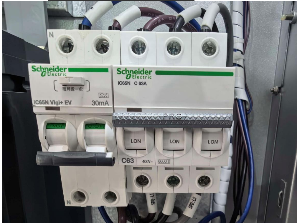
Figure 13 RCD and MCB
