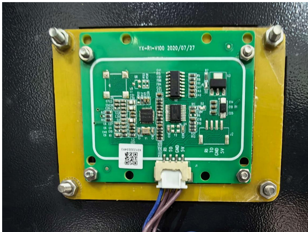
Figure 22 Card reader on the back of the front door
