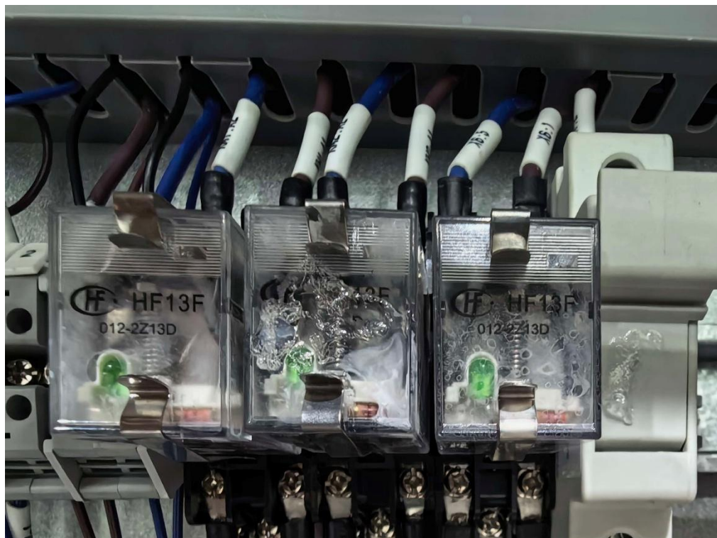
Figure 18 Intermediate relays and AC fuse
