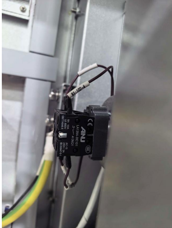
Figure 17 Relay module of emergency stop button
