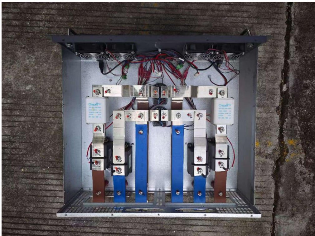
Figure 30 Internal of DC integrated module with SELV cover removed
