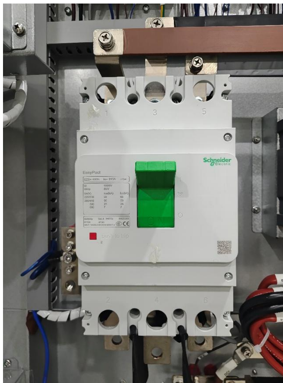
Figure 64 AC circuit breaker QF1
